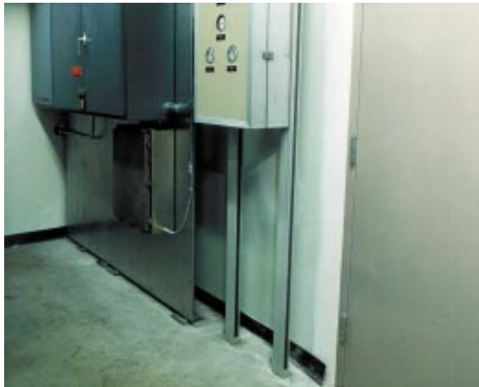
Figure 155: Two different ways to support control panels: using a metal plate attached to floor and ceiling with steel angles (left); using struts extending to floor and ceiling (right).
